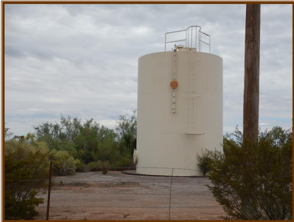
Photo 22. View of larger water tank at the tank site.
